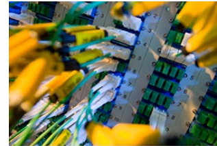
Grid Computing Centre Karlsruhe (GridKa)
